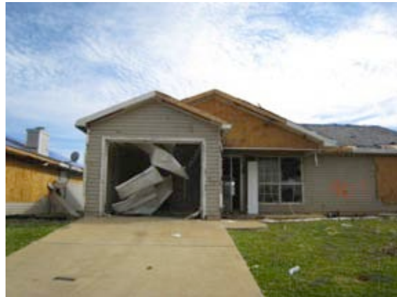
Figure 5.7 Garage wall blown-in
