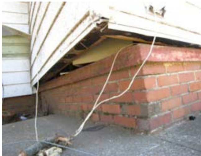
Figure 5.9 House shifting off the foundation
