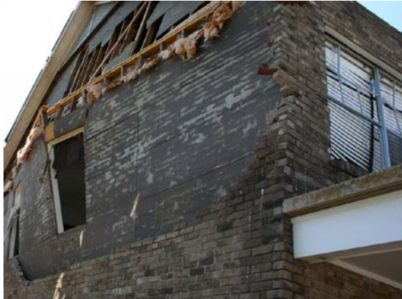
Figure 4.6 Two-story apartment building with gable end failure and brick veneer failure.
