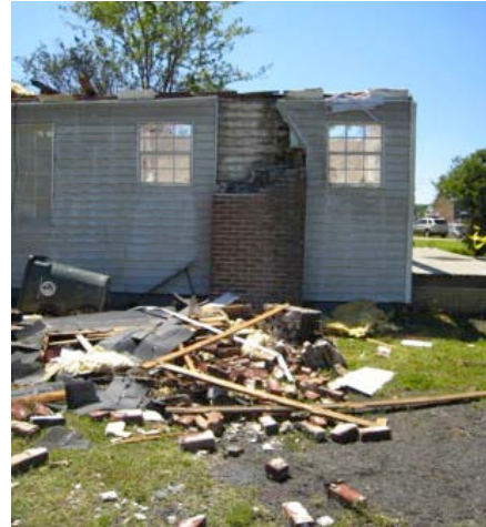
Figure 5.6 Collapse of chimney
