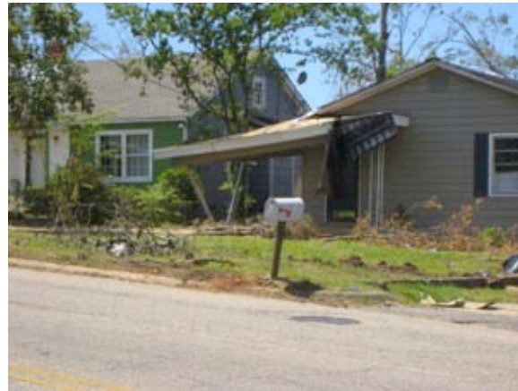
Figure 5.8 Porch or carport damage
