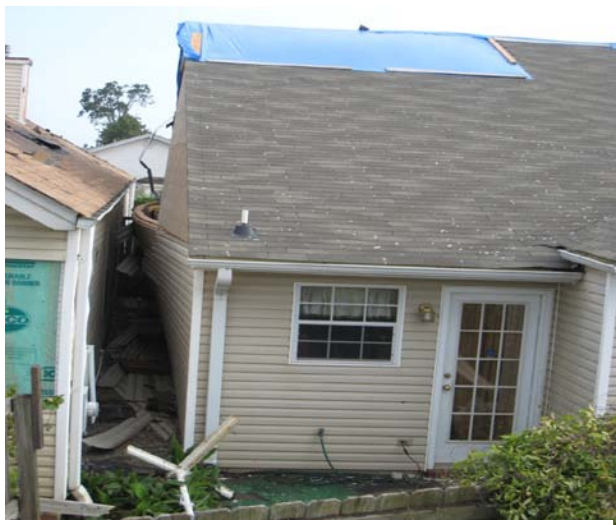
Figure 4.2: Exterior walls pushed out by high internal wind pressure
