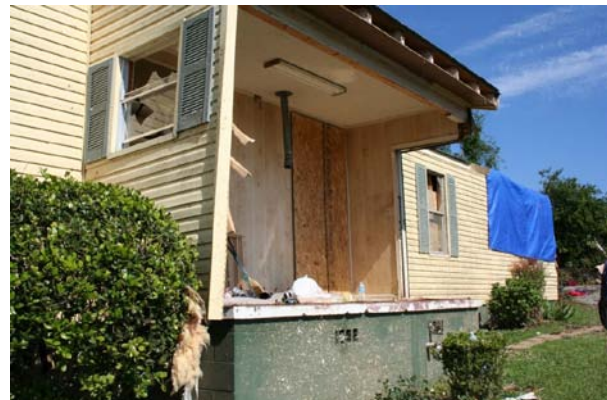
Figure 4.11: Single family dwelling with moderate EF/damage
