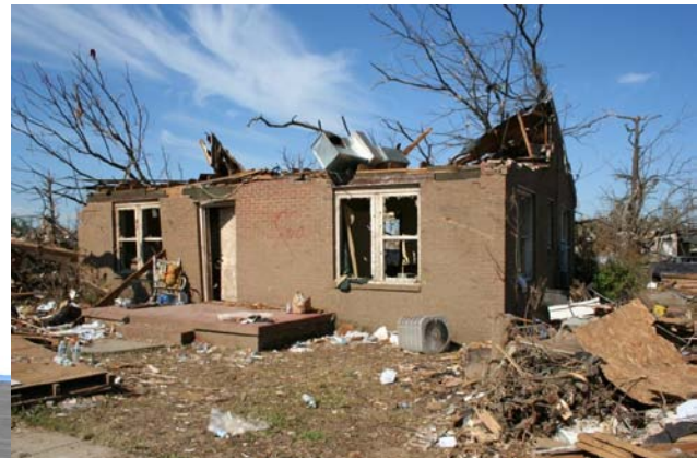
Figure 4.1: loss of roof assembly
