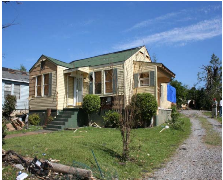
Figure 4.12 Loss of a wall
