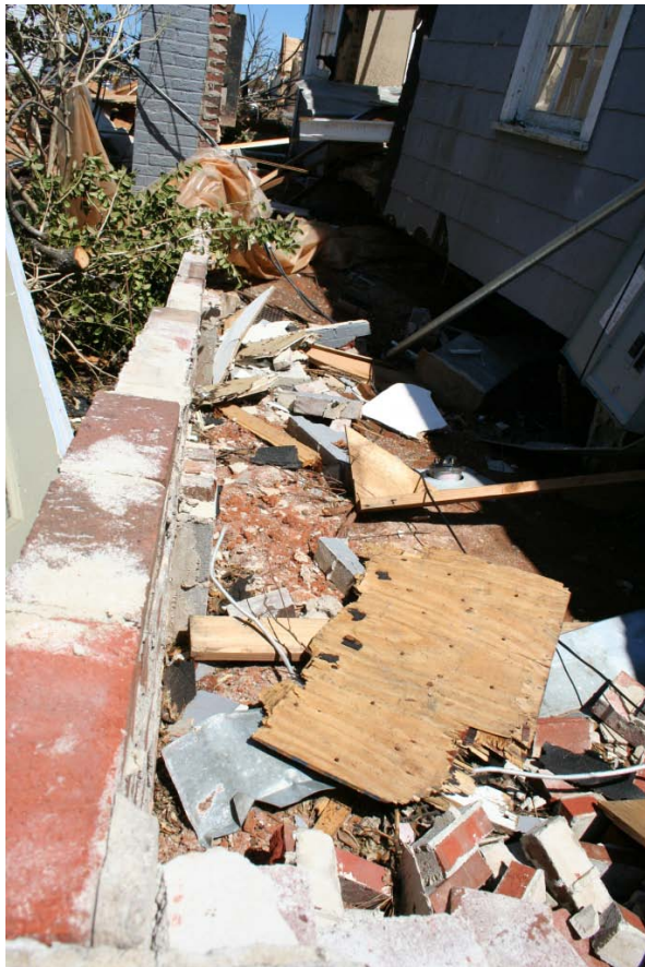
Figure 4.4 House lifted off its foundation. Chimney shown to the right approximately 5ft over.
