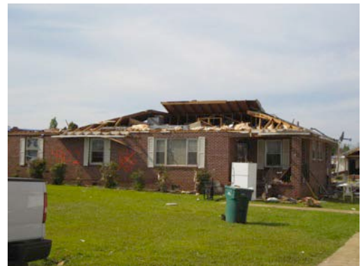
Figure 5.5 Significant roof damage
