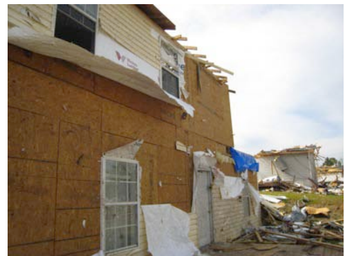
Figure 5.3 Loss of siding material
