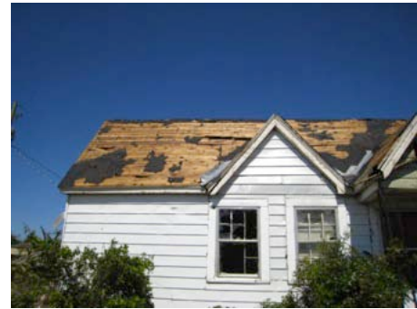
Figure 5.2: Loss of roof covering
