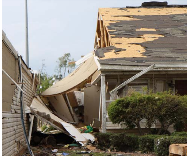
Figure 4.3: Exterior wall and gable roof end pulled out as a result of high leeward winds
