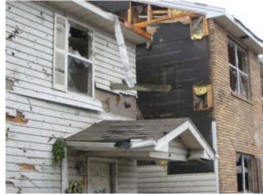
Figure 5.4 Broken windows and doors
