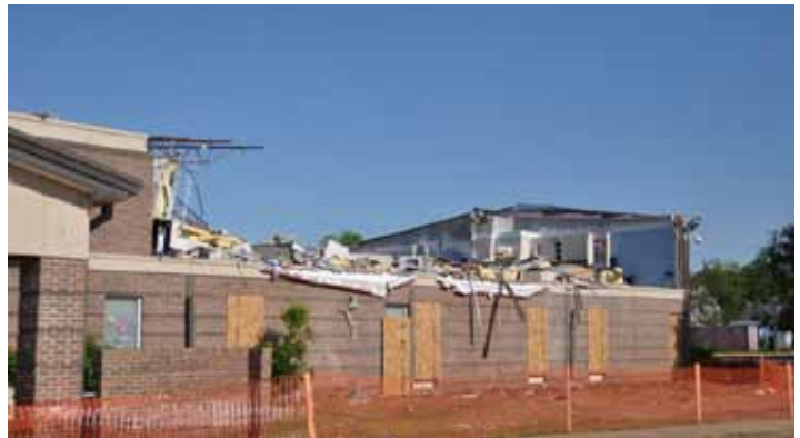
Figure 3: Most of the second floor of one wing collapsed at this 14-year-old school. It had a steel frame with CMU/brick veneer exterior walls.
