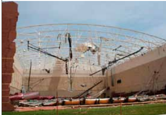
Figure 1: Exterior wall collapsed – no connection at footing
