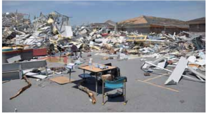
Figure 1: This ten year old one story school had three classroom wings and a central core area. One classroom wing and most of the central core collapsed. This is a view of the central core area.
