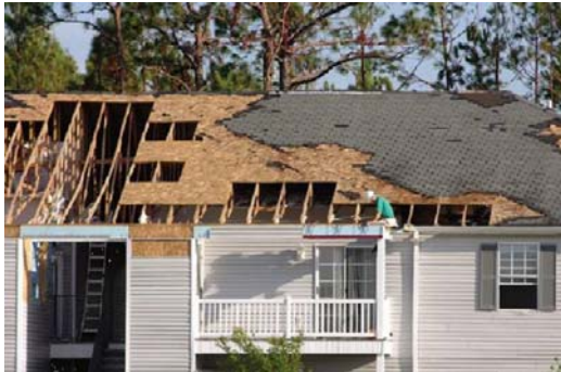
Figure 8. Panel blow-off due to uplift related failures. [FEMA News Photo/ FEMA 549, 2006]
