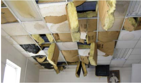
Figure 1. Ceiling collapse due to moisture intrusion after roof membrane failure. [FEMA News Photo/ FEMA 549, 2006]
