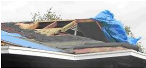
Figure 1: Roof sheathing failures (at ridge and eave) of houses in Hurricane Katrina [9]
